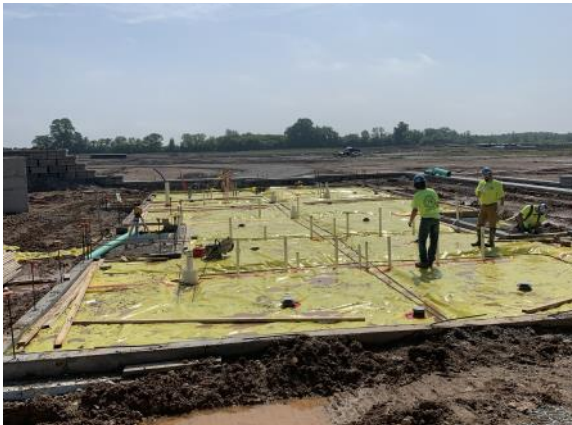
Concrete teams preps for the floor pour in the South concession stand (06/14/2022)
